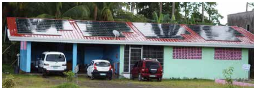
FIRST NET METERS. These solar panels are just part of the total 41,580-watt solar panels installed at one of the buildings in MARIPHIL Children’s Village (Atung Pinuy-Anan) Inc.
