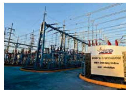
A PIONEER RETURNS. VECO's Don Gil Garcia Switching Station, the utility's oldest substation, was recently upgraded and can now operate more flexibly, reducing operating and maintenance costs.
