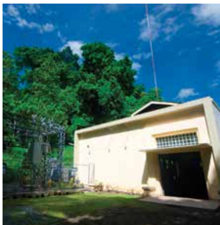
UPGRADED FACILITIES: On-duty plant operator shows the newly installed control panel in Talomo Hydro 3 that's undergoing tests to generate power more efficiently. The plant will be fully automated this November.
