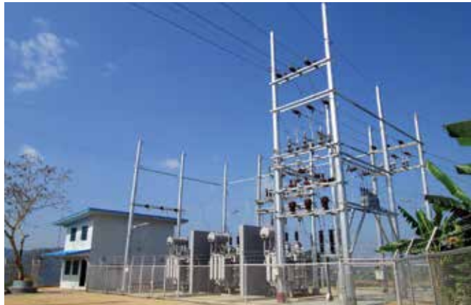
UNINTERRUPTIBLE. The Banengbeng substation's upgraded features ensure steady flow of power supply from generating plants to its customers while state-of-the-art circuit breaker design and switches enable disconnection during inevitable electrical faults and emergency situations and preventing damage.
